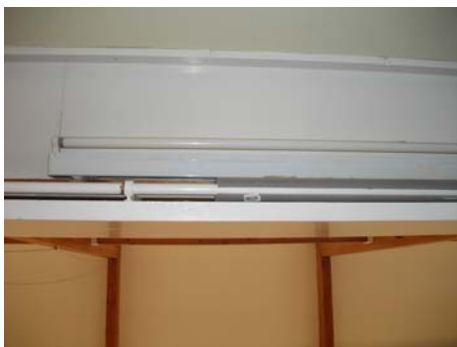
Figure: Strip lighting around main hall perimeter
