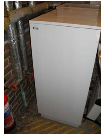
Figure: Floor mounted boiler
