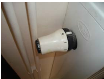
Figure: TRV located on radiator at entrance
