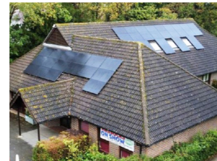
Solar panel arrays on the roof combined with internal battery storage.
